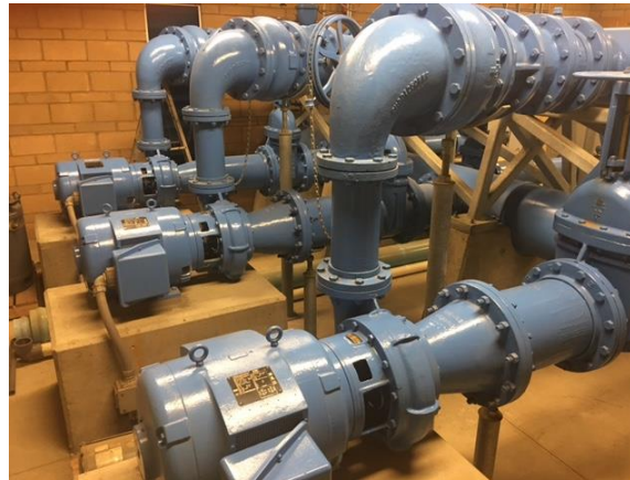
City of Guadalupe Obispo Boosting Station
